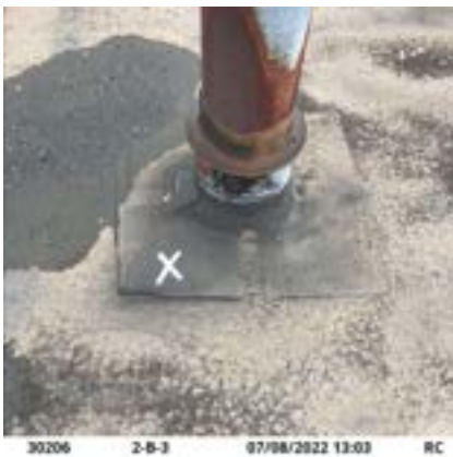
Deteriorated penetration flashing. Insulation is saturated with water around this penetration.
