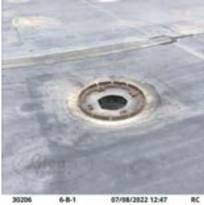
Missing drain basket
