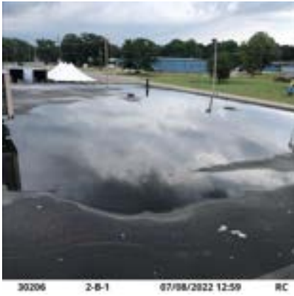
Large areas of ponding water due to lack of slope.
