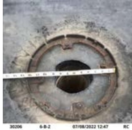
Missing drain basket
