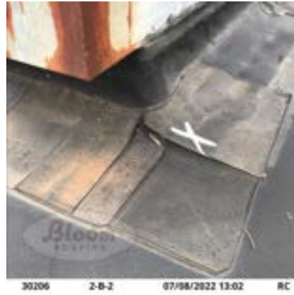
Lifting and open corner flashing
